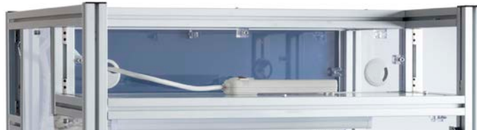
Integrated power strip provides a convenient and accessible location for valve controller installation.
