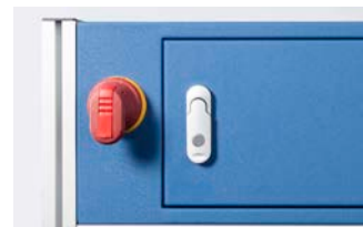
Main disconnect switch
