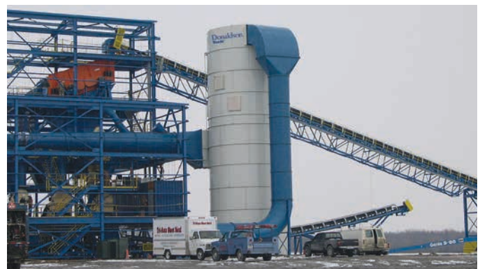
780LP12 at Coal Classifying Plant 75,000 cfm (127,339 m 3 /h)
