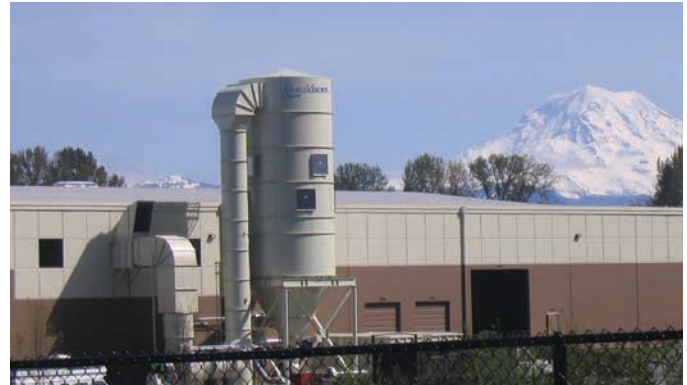
528LP12 at Cabinet Factory 70,000 cfm (118,906 m 3 /h)
