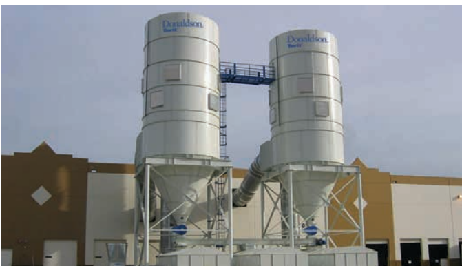
TWO 594LP12 at Cabinet Plant 80,000 cfm/each (135,892 m 3 /h each)
