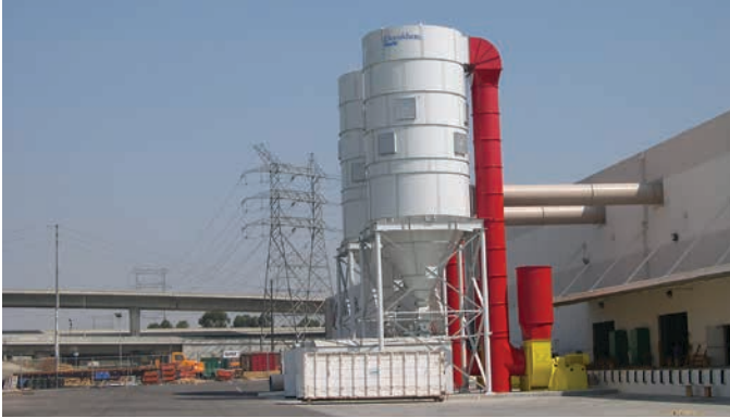
Dual 594LP12 at Door Plant 180,000+ cfm/combined (305,757+ m 3 /h combined)
